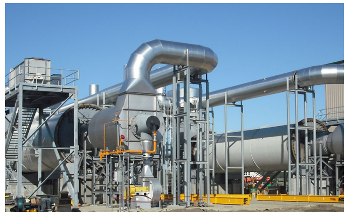
Typical high capacity rotary drier installation for industrial applications.
